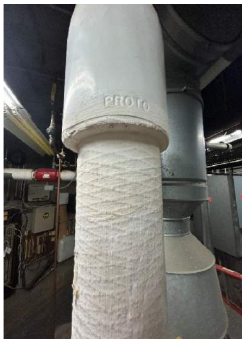
Photograph 3: HID 02. Pipe Endcap Mastic (NAD)
