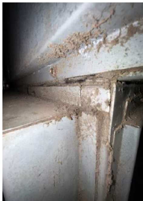
Photograph 4: HID 03. Black Air Handler Unit Caulk (NAD)
