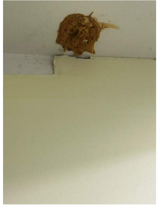
Photograph 14: HID 15. Glue Dots (NAD) associated with smoke detectors.
