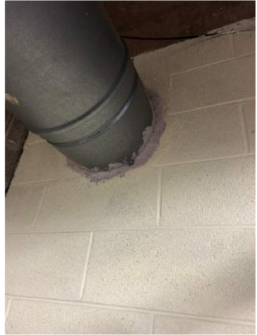
Photograph 6: HID 05. Flue Packing (NAD)
