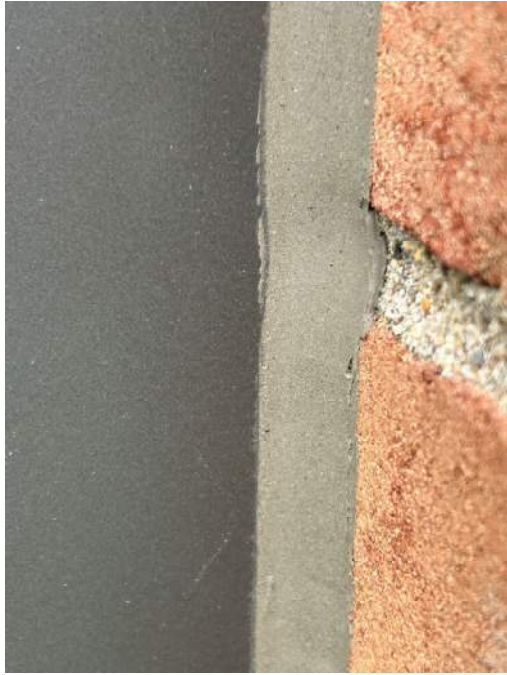
Photograph 13: HID 14. Exterior Window Caulk (NAD)
