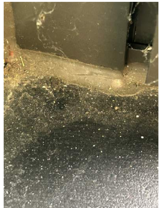
Photograph 12: HID 13. Interior Window Caulk (NAD)
