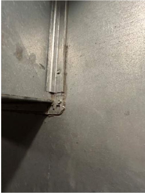
Photograph 5: HID 04. Gray Air Handler Seam Caulk (NAD)
