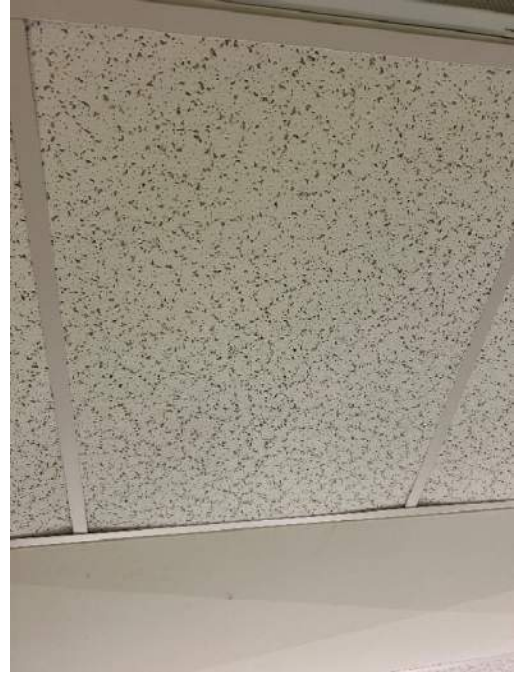
Photograph 10: HID 10. 2'x4' Dot Fissure Ceiling Tile (NAD)
