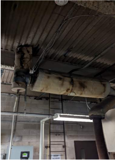
Photograph 2: HID 02. Generator Thermal Insulation (NAD)
