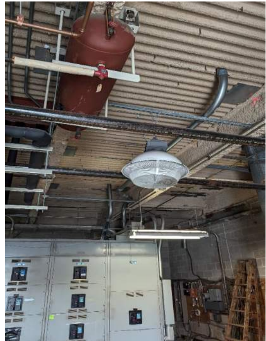
Photograph 52: Mercury Light Fixture
