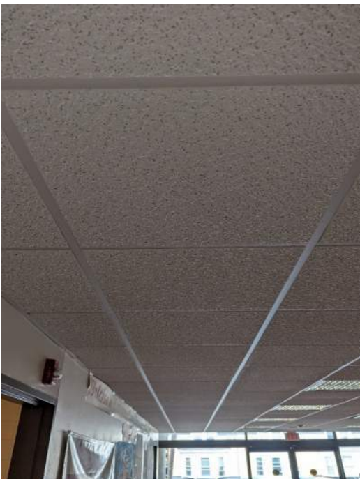
Photograph 26: HID 37. 2'x2' Ceiling Tile (NAD)
