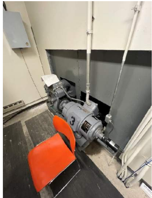
Photograph 56 Elevator Gear System on 2 nd Floor
