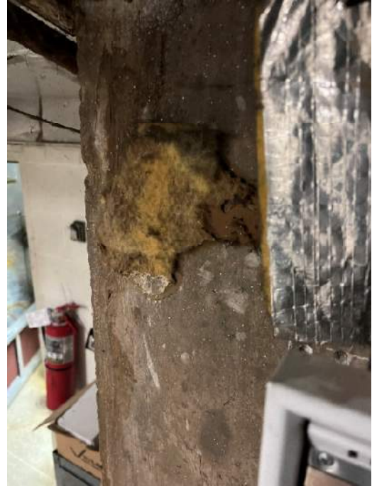
Photograph 42: HID 48. Glue Dots (NAD) associated with Fiberglass Panels
