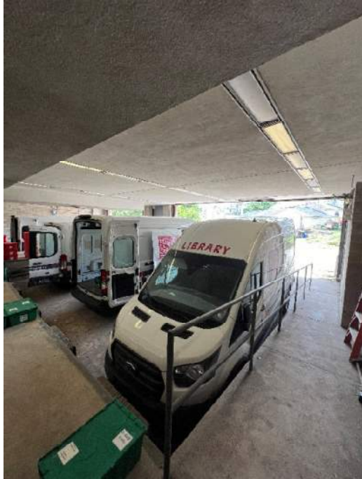
Photograph 41: HID 30. Ceiling Plaster (NAD), In Garage
