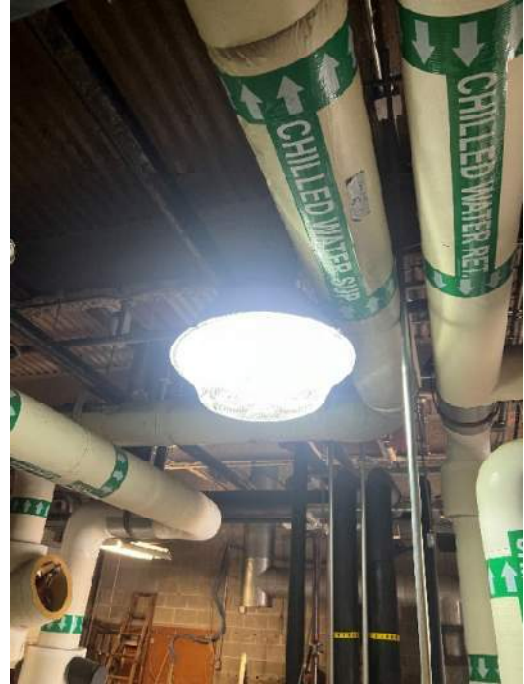
Photograph 50: Mercury Light Fixture
