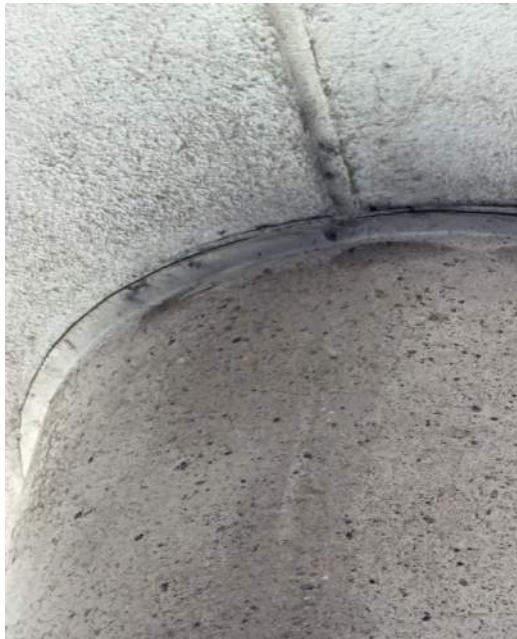
Photograph 35: HID 49. Exterior Plaster Ceiling Expansion Caulk (NAD)
