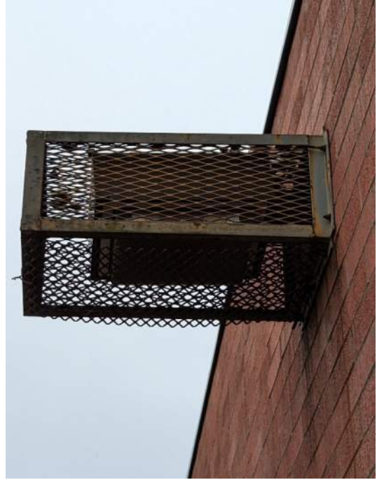
Photograph 54. Exterior Mercury Light Fixture
