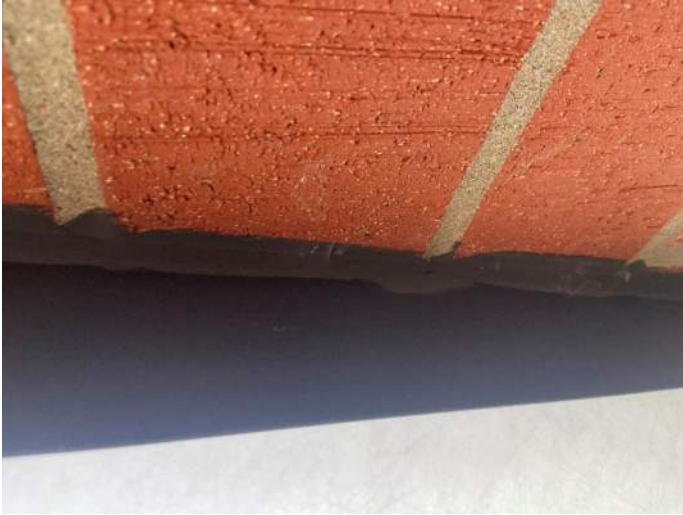
Photograph 13: HID 21. Interior Window Caulk (NAD)
