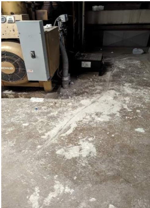
Photograph 3: HID 02. Generator Thermal Insulation (NAD) Debris on Floor
