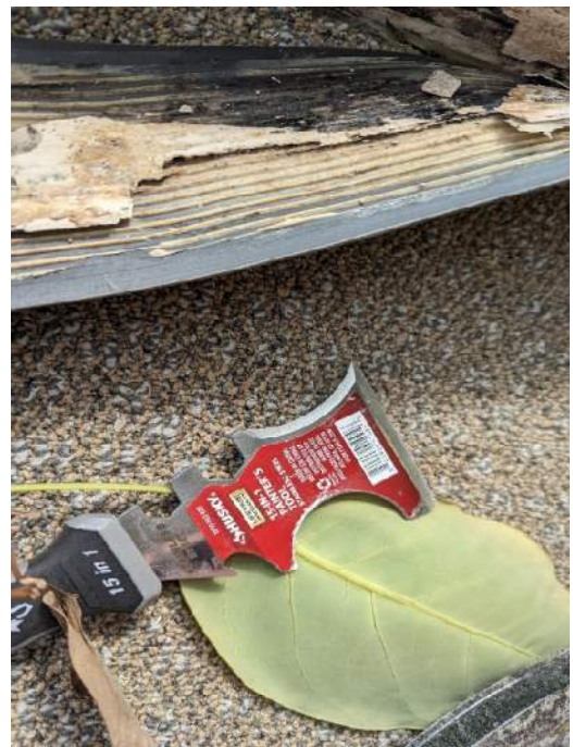
Photograph 24: HID 35. Covebase Mastic (NAD)
