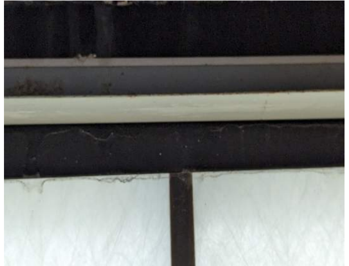
Photograph 22: HID 33. Interior Window Caulk White (NAD)
