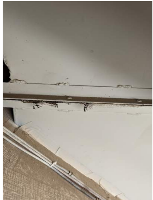
Photograph 8: HID 07. Duct Seam Caulk (ACM)
