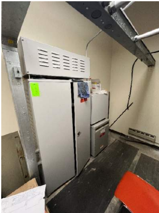
Photograph 55: Dry Transformer – 2 nd Floor, Elevator Room
