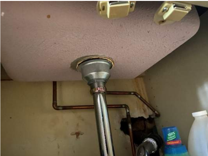
Photograph 19: HID 29. Pink Sink Undercoating (ACM)
