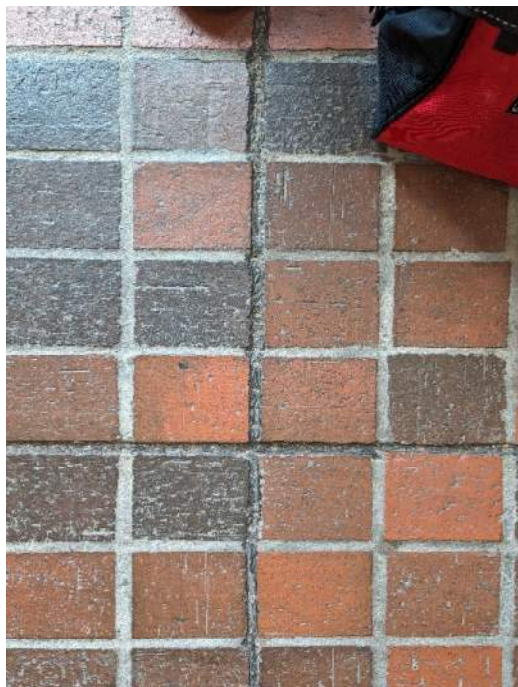
Photograph 27: HID 38. Brick Floor Expansion Caulk (NAD)
