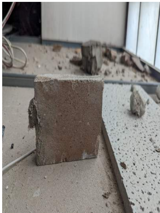
Photograph 10: HID 10. 2'x4' Dot Fissure Ceiling Tile (NAD)
