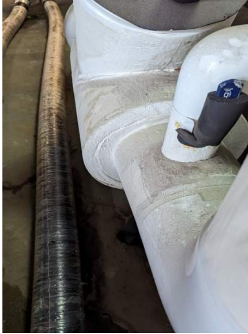
Photograph 5: HID 04. Endcap Mastic (NAD)
