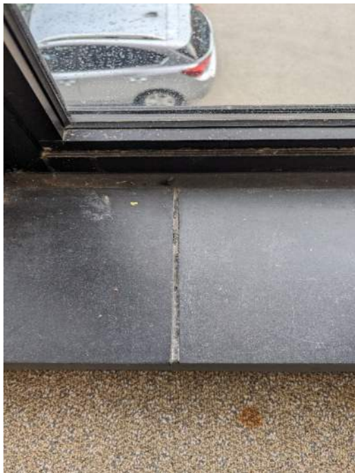
Photograph 23: HID 34. Interior Window/Ledge Black Caulk (NAD)
