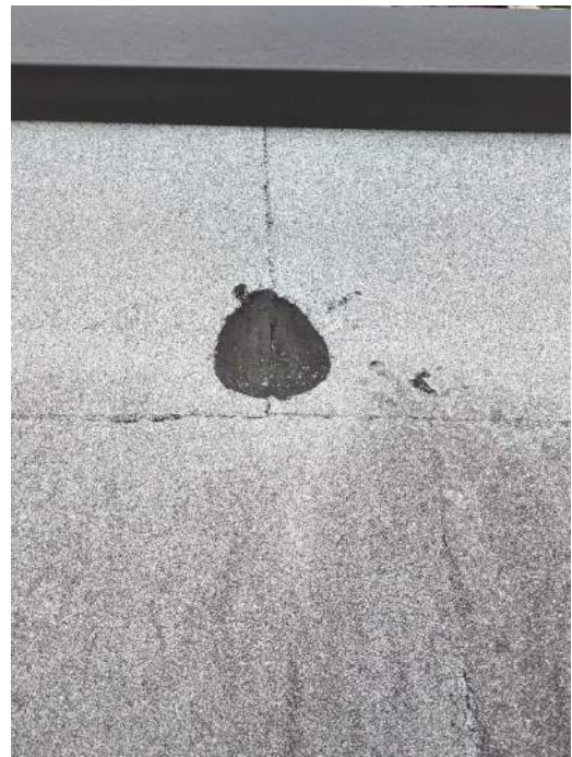
Photograph 44: HID 43. Roof Seam Tar (Not Sampled/Presumed ACM)
