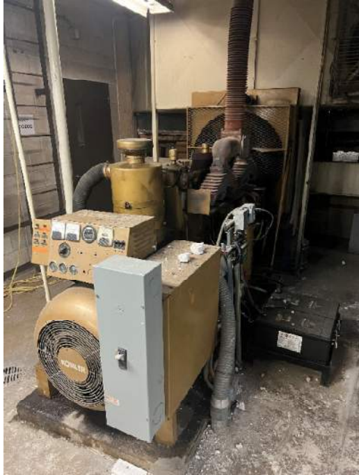
Photograph 49: Natural Gas Generator
