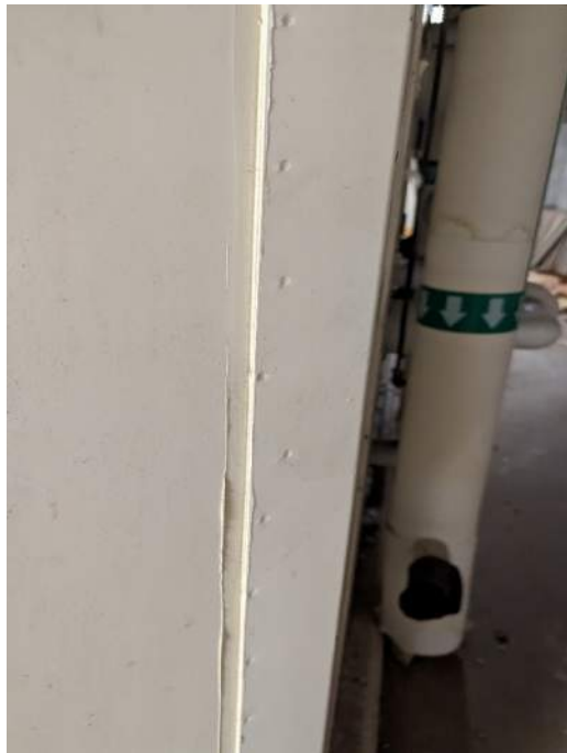
Photograph 7: HID 06. Air Handler Caulk (ACM)
