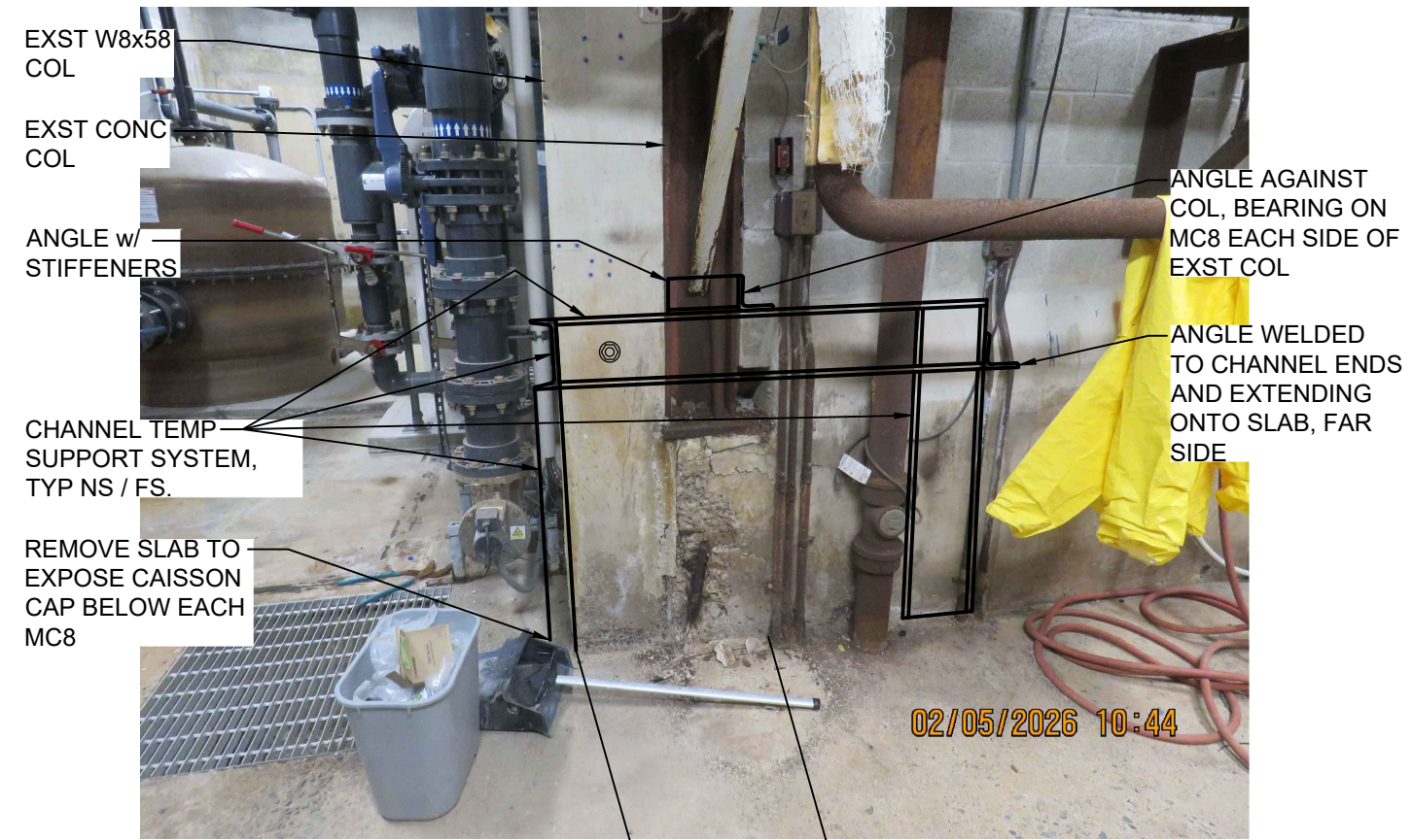
8 REFERENCE PHOTO S502 SCALE: NONE PHOTO SHOWN FOR BASIC COLUMN SHORING INTENT AND REFERENCE ONLY. SEE DETAILS ON THIS SHEET FOR ADDITIONAL INFORMATION, COMPONENTS, SECTIONS AND DETAILS RELATED TO SHORING
